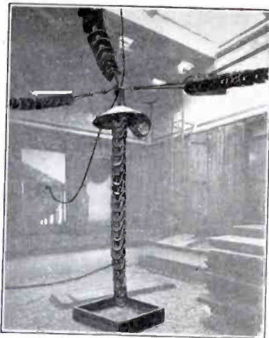
Striking View of the Large Lead-In Insulators Which Are Located in the Small Court-Yard Immediately in the Center of the Station.
